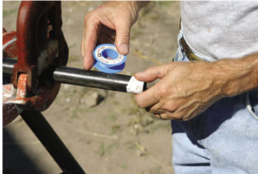
Teflon tape or pipe thread sealing compound is placed on the threads.
