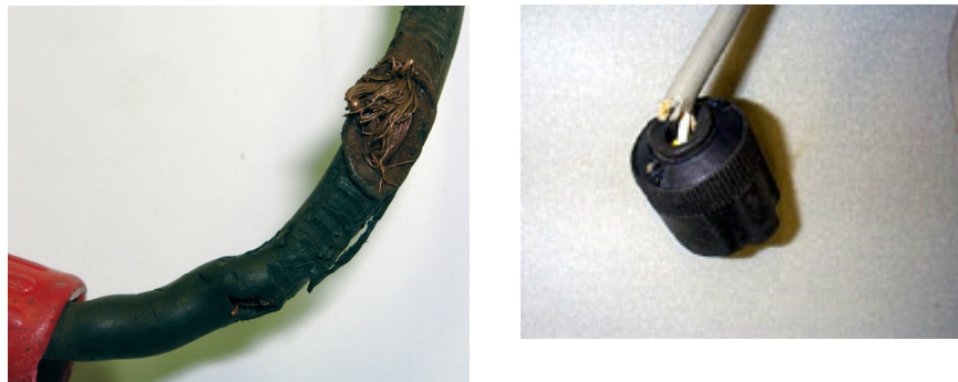
Figure 14—Frayed cables and strained cables caused by inappropriate use
